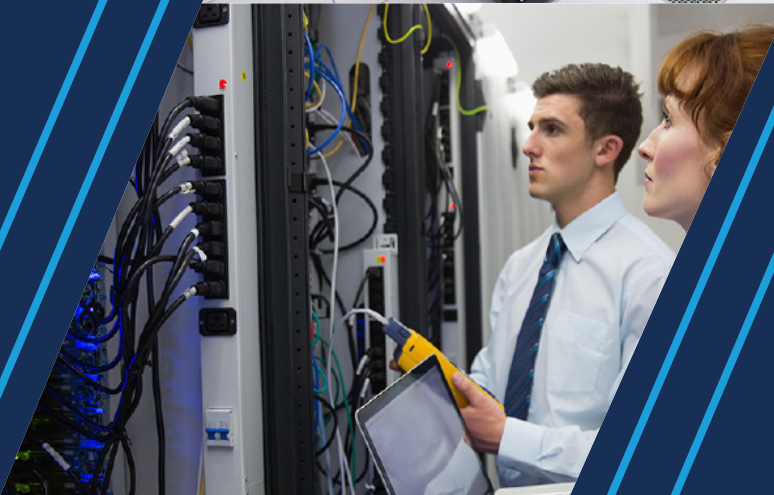
Data Center System
